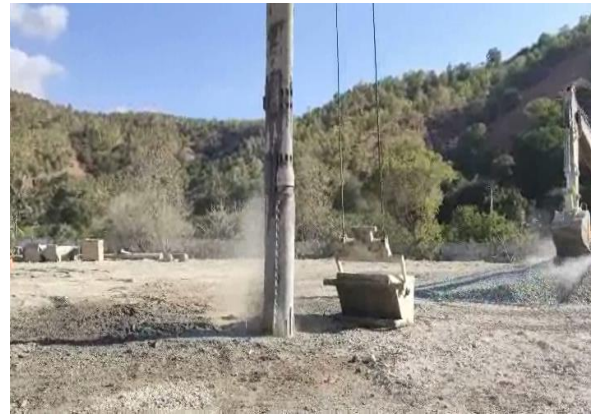
图 6 东帝汶帝力帝巴湾新集装箱码头干法底部出料振冲施工 Fig. 6 Bottom feed vibroflotation dry construction in Timor-Leste Dili new container port project
