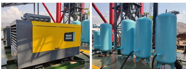
图 5 干法底部出料振冲施工配置的空压机和空气储气罐 Fig. 5 Air compressor and air accumulator for bottom feed vibroflotation dry construction
