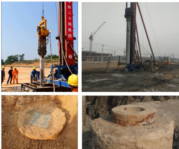
图 4 大直径超深搅拌加芯一体化桩机施工现场 Fig. 4 Construction site of large diameter ultra-deep mixing and core integration pile machine
