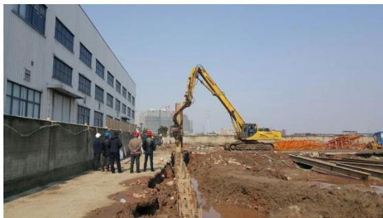
图9 帽型H型钢组合钢板桩的施工 Fig. 9 Construction of H+Hat combined steel sheet pile
