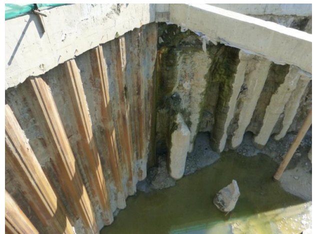
图4 挡土墙止水性比较 Fig. 4 Comparison of water retention of retaining walls
