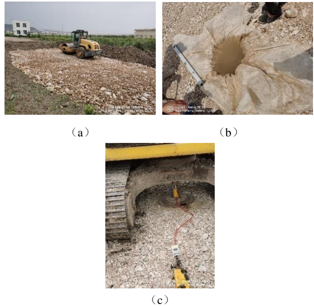
图 2 现场碾压施工和灌水法、承载板法的检测 Fig. 2 In-situ rolling construction and inspection of irrigation method and bearing plate method
